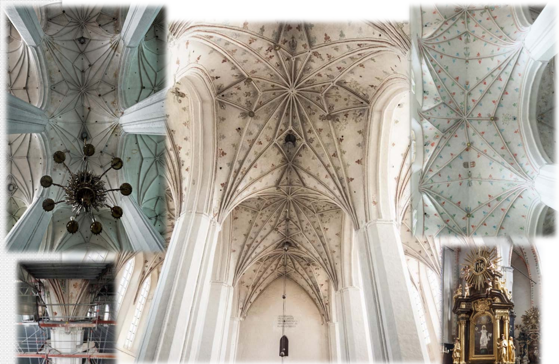
Cathedral Parish Church of St. John the Baptist and St. John the Evangelist: the restoration of the painted vaults, walls, altars, epitaphs, chapels
